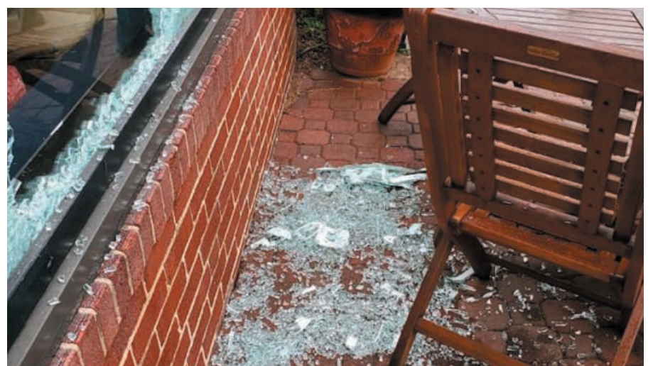
Damage done to the front of Social Coffeehouse. Photo credits: Lisa Kotyk, owner of Social Coffeehouse
