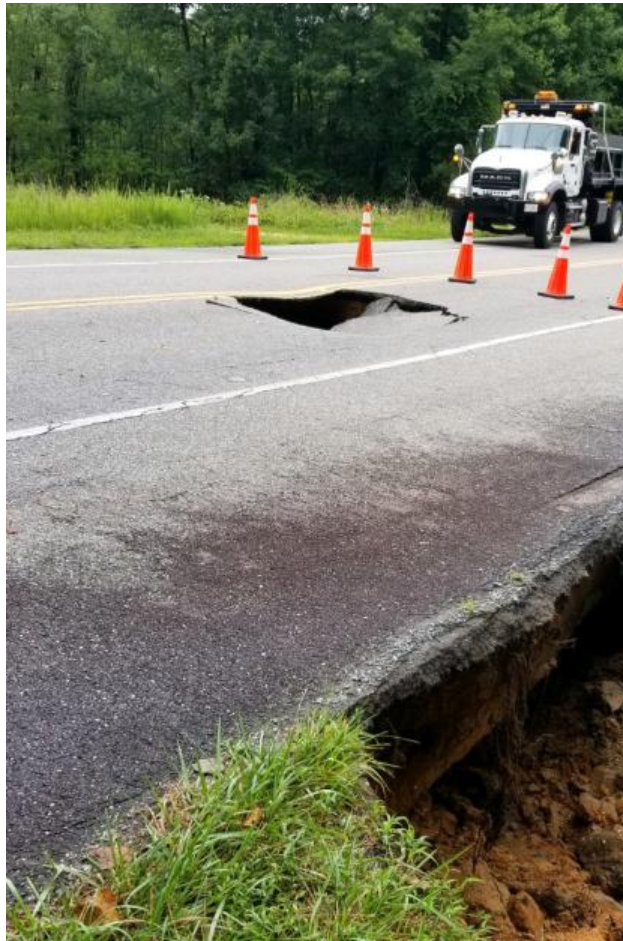
Cox Road's culvert collapse due to heavy rains.
