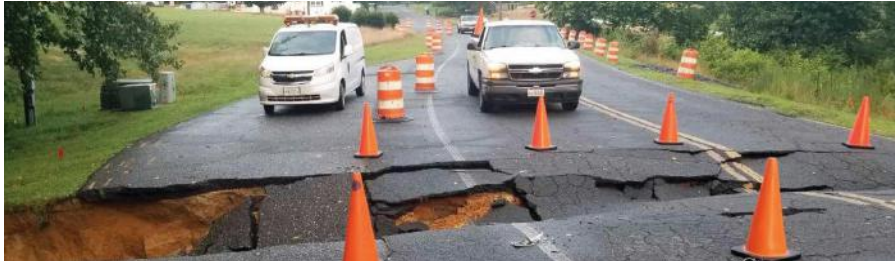
Moakley Street after being washed out.
