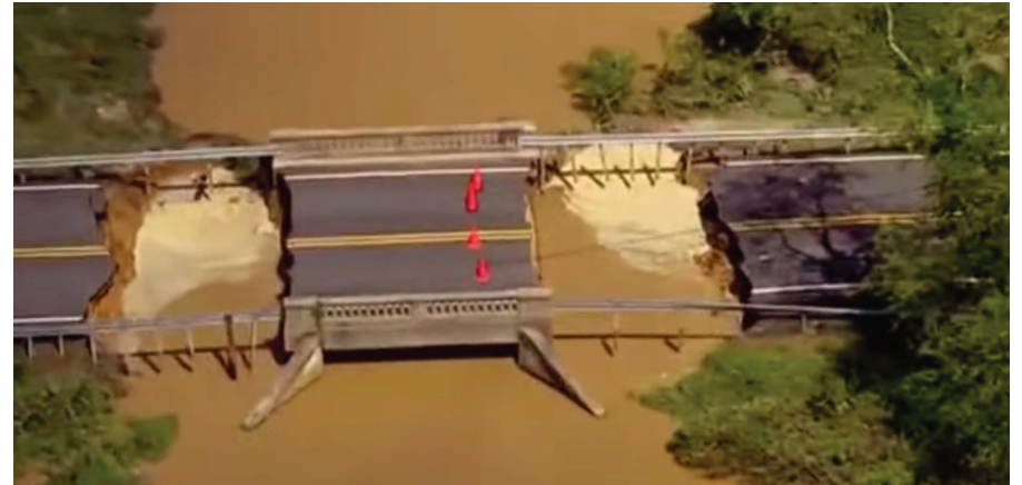
The bridge over Persimmon Creek after being washed out Aug. 4.
