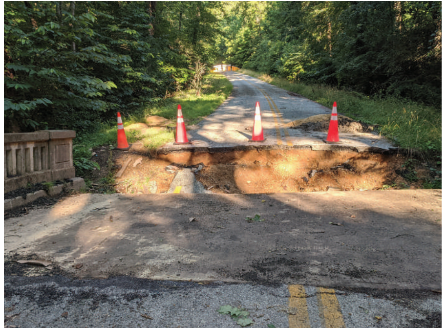
Manor Bridge Road washed out.
