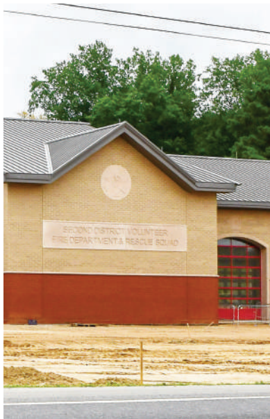
FIRE DEPARTMENT 17 The new Valley Lee fire house should be completed this fall.
