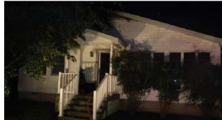
LOCAL 6 Fire damages Lusby home
