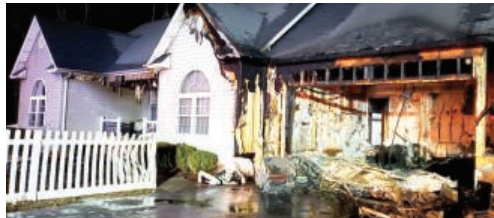
18 LOCAL 8 Huntingtown fire started in garage.
