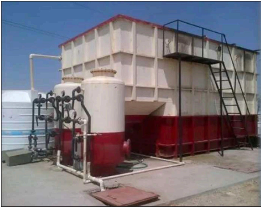
An example of a package plant for waste water treatment
